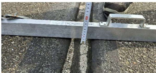
-: opening (spleet) in asfalt
